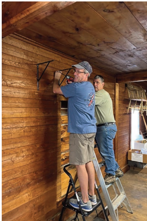
Brad Stevens and his neighbor Rick Nichols work on the dining room wall after moving the shelf units to the third floor.
