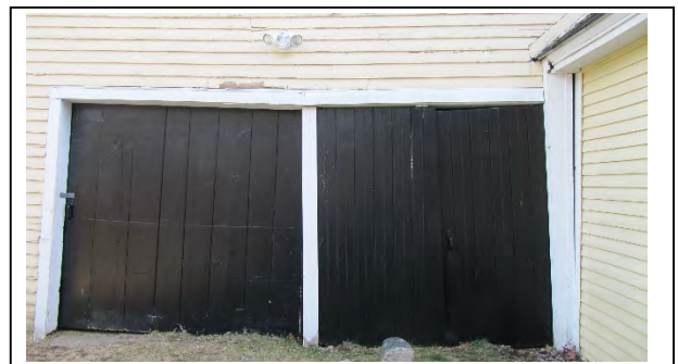
The door wall, buckling in the middle and moved off its sill.
